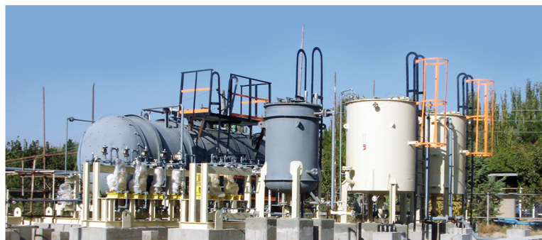
Neutralization package of Tabriz Refinery
