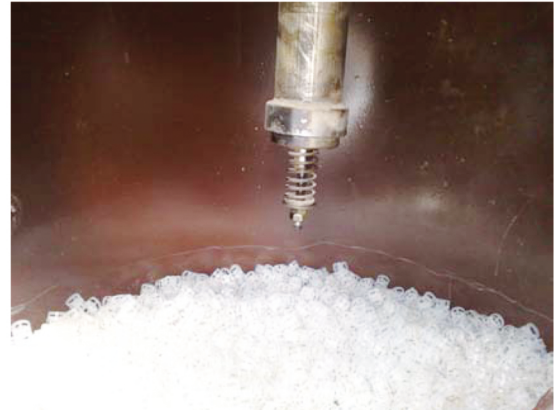
First Stage of Vacuum Deaerator Tower Spray Valve and Packing Bed
